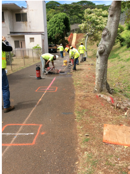
Preparing for augering and fence post installation through the existing access road.
