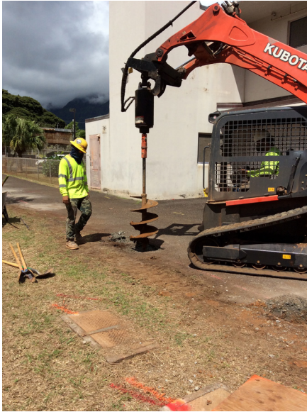
View of augering through existing asphalt pavement for temporary security fence installation
