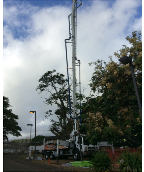
Concrete pump truck used for concrete pour of security fence grade beams.
