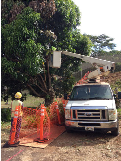
Tree pruning process commenced near Kaala Cottage to meet clearance for the temporary security chain-link fence.
