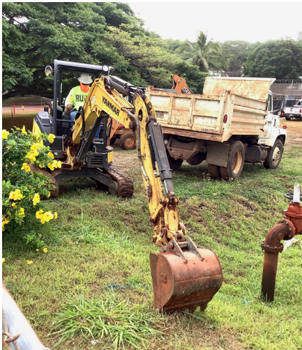
Excavation for the temporary water line commenced near the main entrance and backflow preventer.
