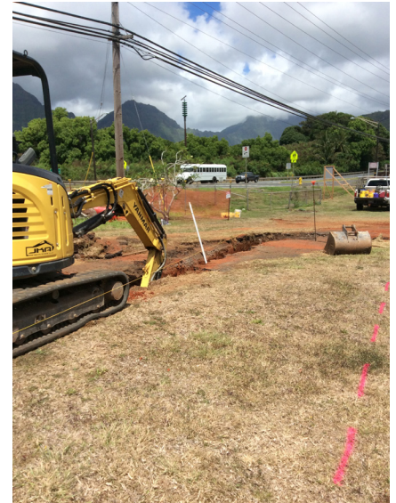
Excavation underway for temporary sewer line. Once installed, sewer line is then backfilled and compacted using a rolling compactor.
