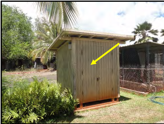
HM ID: 111 Electrical Shed Floor 1
