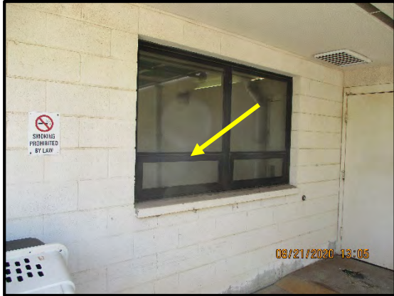
HM ID: 89 Admin Building Floor 1 Exterior Black paint on metal door. Assumed LCP (Baked on paint)
