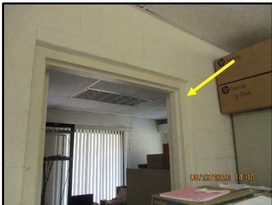
HM ID: 182 Admin Building Floor 2 Office 1 White paint on metal door frame. Non-LCP 2819-B-P76A: <40 mg/kg 2819-B-P76B: <40 mg/kg
