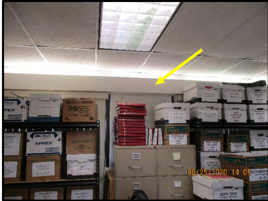
HM ID: 180 Admin Building Floor 2 Office 1 White paint on drywall wall. Non-LCP 2819-B-P74A: <40 mg/kg 2819-B-P74B: <40 mg/kg
