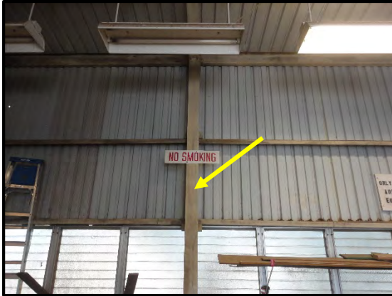
HM ID: 218 Maintenance Shop Floor 1 Warehouse Off-white paint on metal H-beam.
