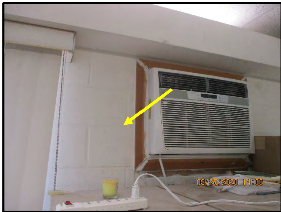
HM ID: 181 Admin Building Floor 2 Office 1 White paint on concrete block wall. Non-LCP 2819-B-P75A: <40 mg/kg 2819-B-P75B: <40 mg/kg
