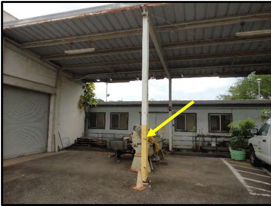
HM ID: 201 Maintenance Shop Floor 1 Exterior Yellow paint on metal corner trim.
