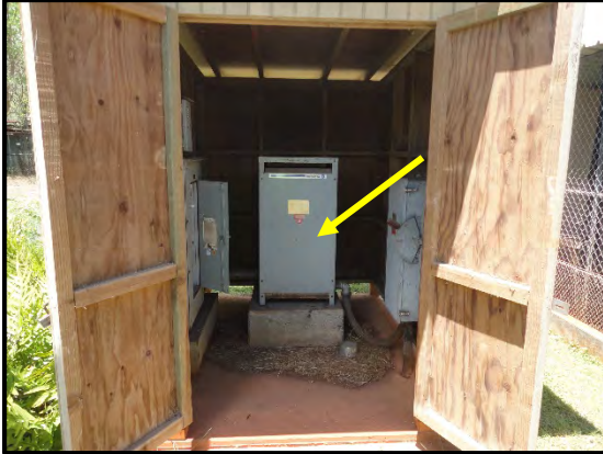
HM ID: 110 Electrical Shed Floor 1
