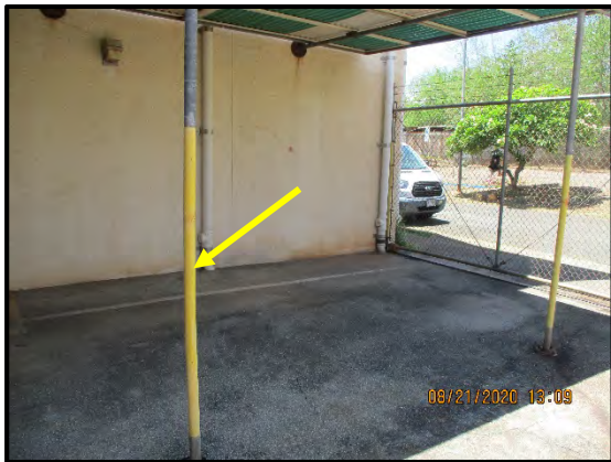
HM ID: 90 Admin Building Floor 1 Exterior Yellow paint on pole. LCP 2819-B-P55A: 530 mg/kg 2819-B-P55B: 550 mg/kg
