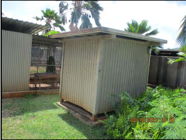
Electrical Sheds August 2020
