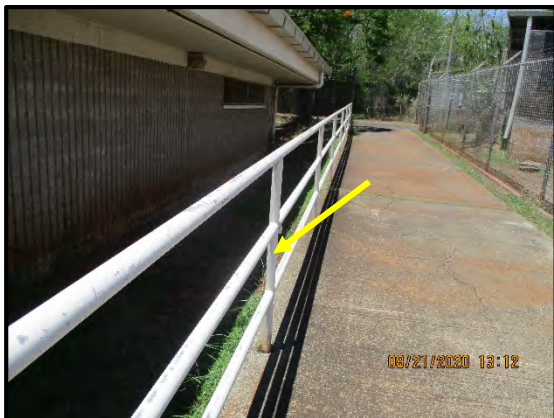
HM ID: 91 Admin Building Floor 1 Exterior White paint on metal railing. LCP 2819-B-P56A: 490 mg/kg 2819-B-P56B: 500 mg/kg
