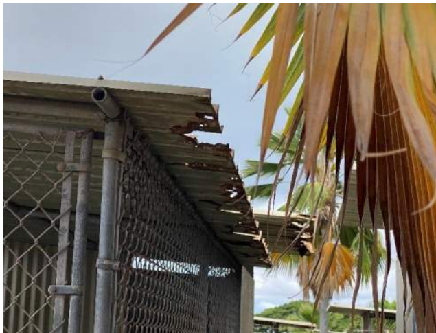
Photo-46: Rust at the Metal Roofing
