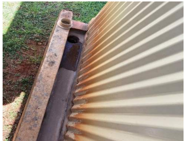
Photo-47: Rust at Metal Walls and Drain
