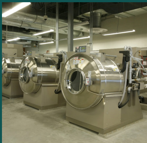
Representative Laundry Operation
