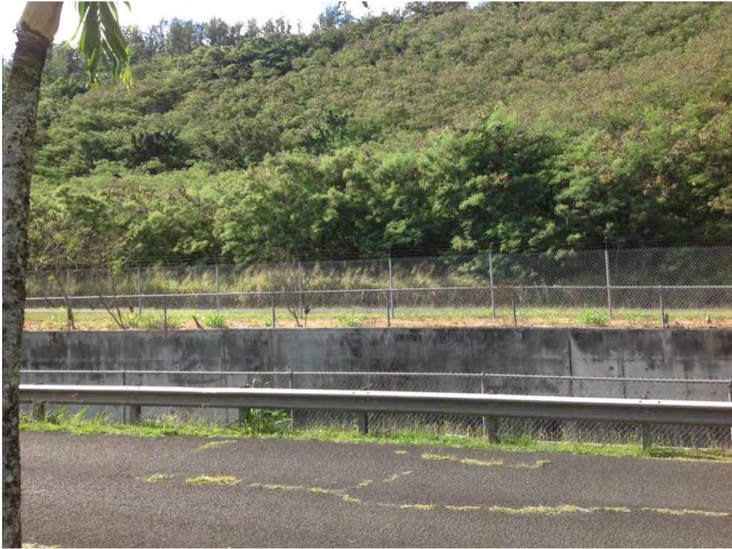
Photograph 3: View looking southeast at southern property boundary showing concrete lined channel and steep slope of adjacent property
