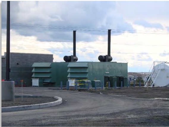
Emergency Generator Example
