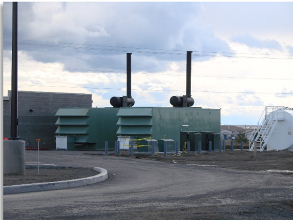
Emergency Generator - Example
