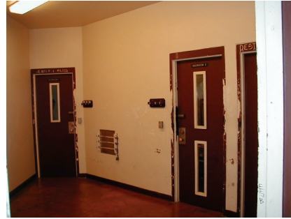
Example of building maintenance/repair needs - Kauai Community Correctional Center
